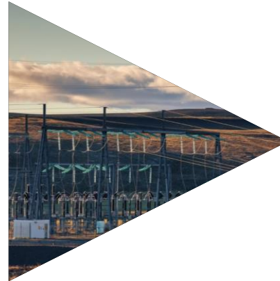
Electrical Power Supply Networks
